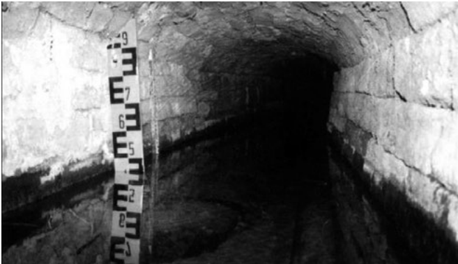
Fig. 4: Mine water as a geothermal potential – inside the "Froschmulden" drainage tunnel/district Mansfeld-Südharz (Photo: BdU)
